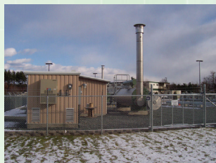
Metering and Regulating Station
